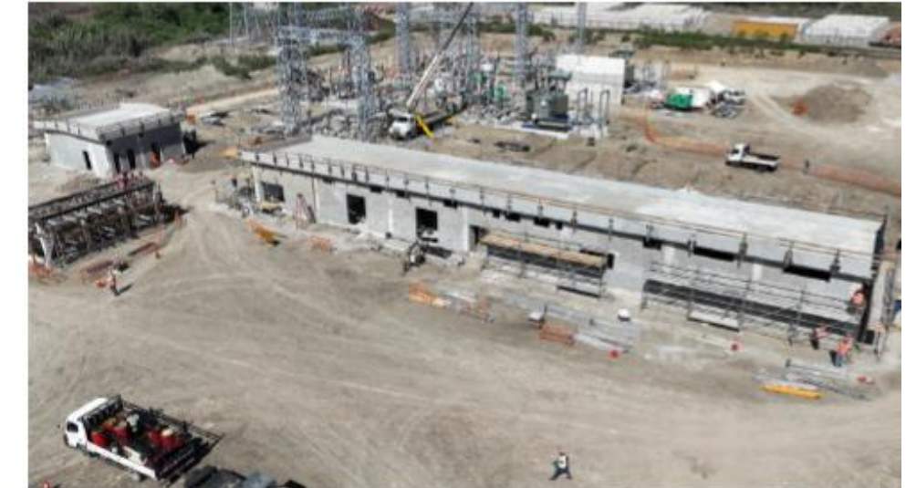
SS - CONTROL BUILDING
